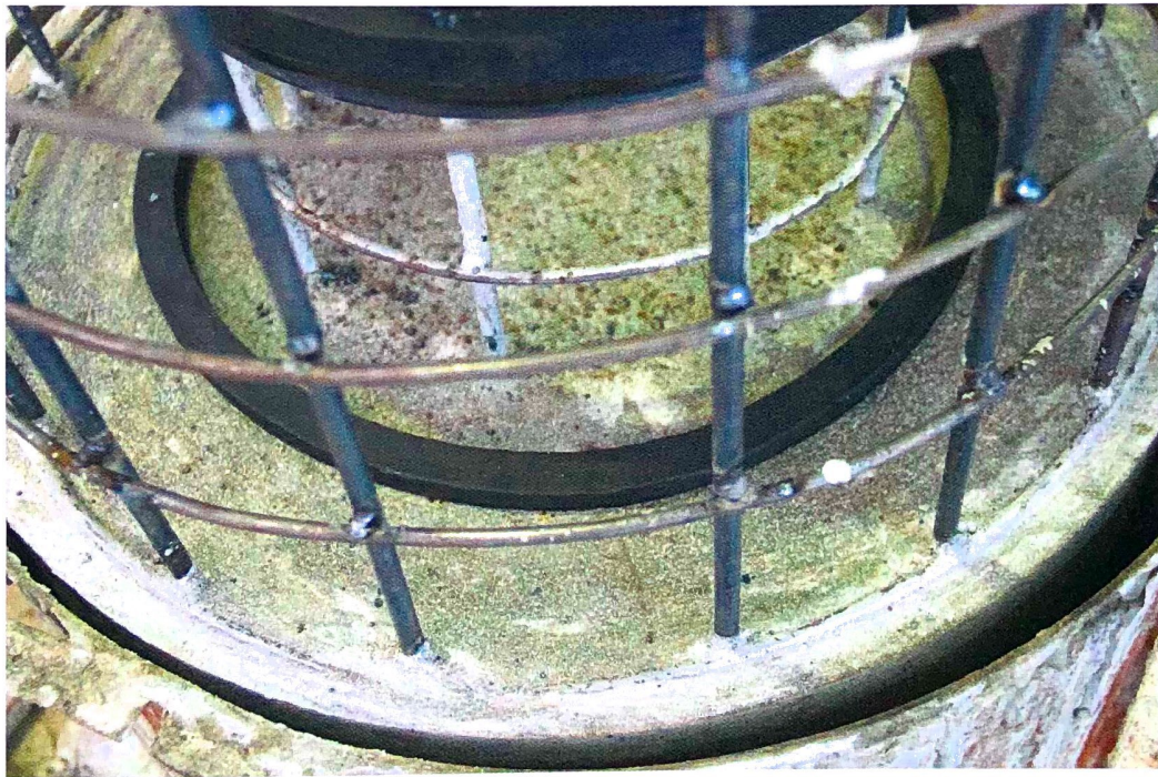
Photograph 2 – Installation of RHINOSWELL Swelling Waterstop (20x15 mm) along the construction joints of the concrete test chamber.
