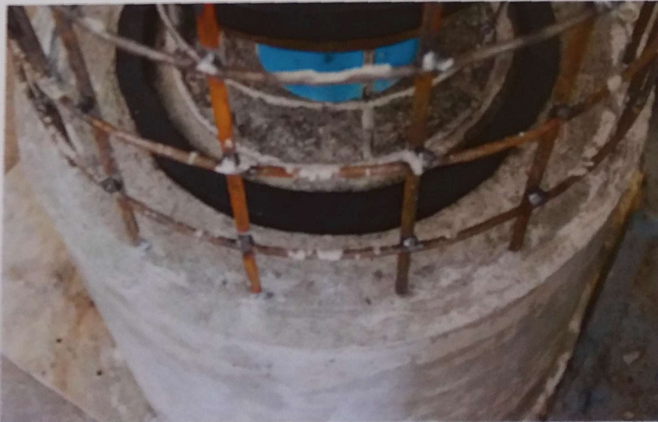
Photograph 2 – RHINOSWELL waterstop installed along the construction joint of the concrete test chamber
